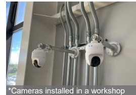
*Cameras installed in a workshop
